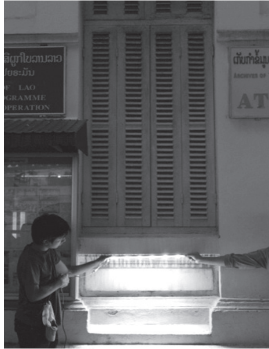
LED 12.6W – downlighting
