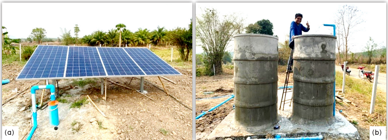
Figure 5 (a) Bamboo garden water supply system and (b) Water tank
