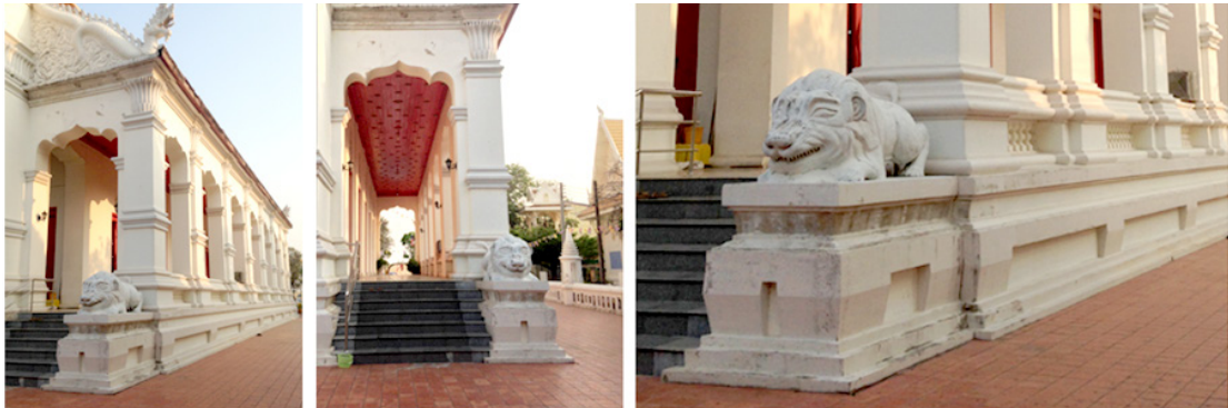
Figures 16-18 Stairway, foundation elements, lion sculpture and corridor passage of the ordination hall, Wat Supattanam
